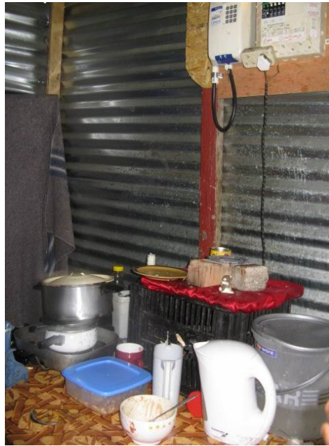
Fig. 5: Anonymous respondents described waiting eight months prior to being connected to the City of Cape Town's electricity grid. Connections are precarious and unsafe. Water seeps through the roofs of some of the shelters and consequently electrical shorts occur due to exposed electrical connections. Various homes have burnt down as a result.
