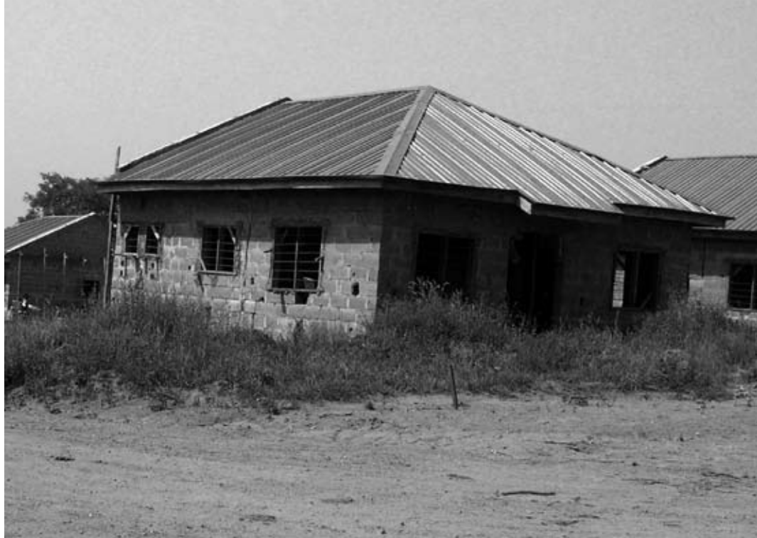
Apo resettlement site: poorly constructed housing [Photo: Deanna Fowler, Dec. 2006]
