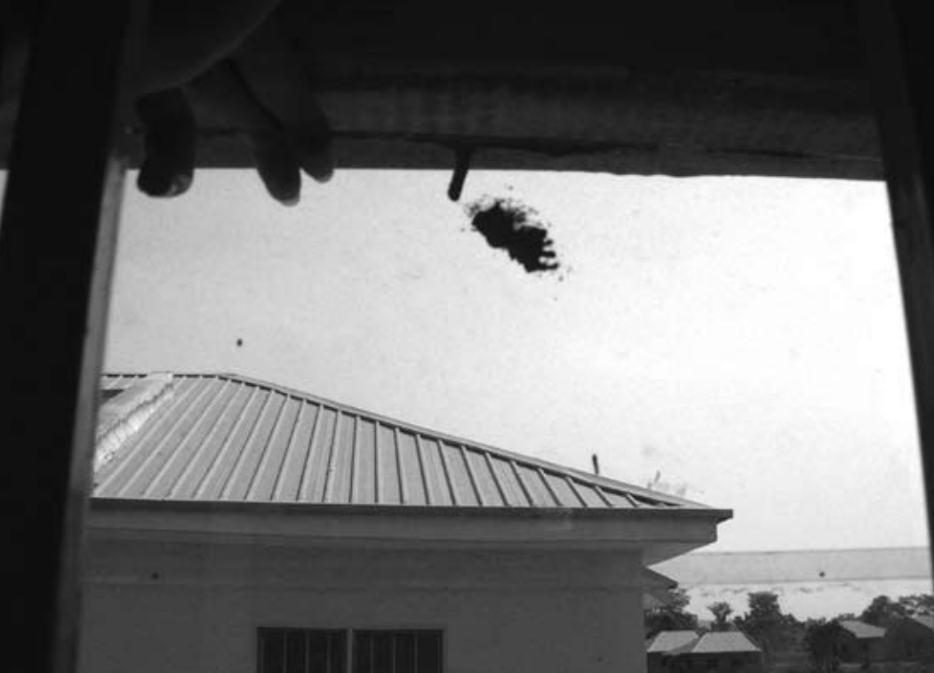
Windows do not fully shut, allowing open space of several centimeters [Photo: Deanna Fowler, Dec. 2007]
